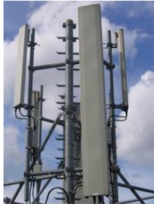
▼ ANTENNE TELECOM (PAM PRO)
